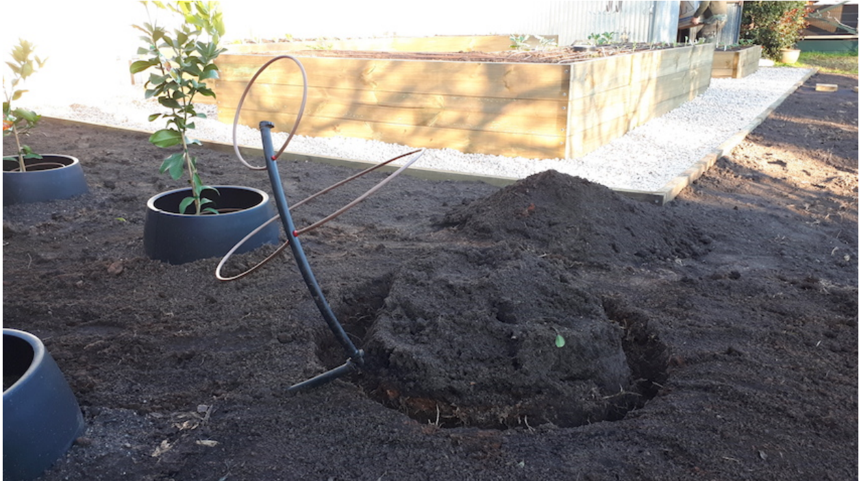
A rather odd looking irrigation pipe. It will eventually be laid flat over the mound where pumpkins and melons will be planted.
